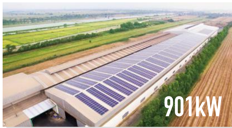
Project Type: Commercial Rooftop Location: Thailand / Chachoengsao Commission Date: 2018-1 Product: SRP-340-6MA
