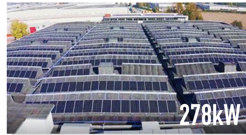
Project Type: Commercial Rooftop Location: Italy / Dalmine (BG) Commission Date: 2020-5 Product: SRP-315-6MB
