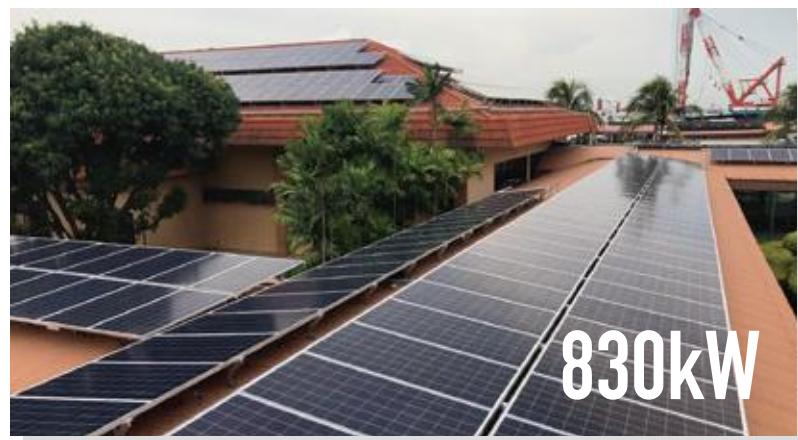
Project Type: Commercial Rooftop Location: Singapore Commission Date: 2017-10 Product: SRP-325-6PA
