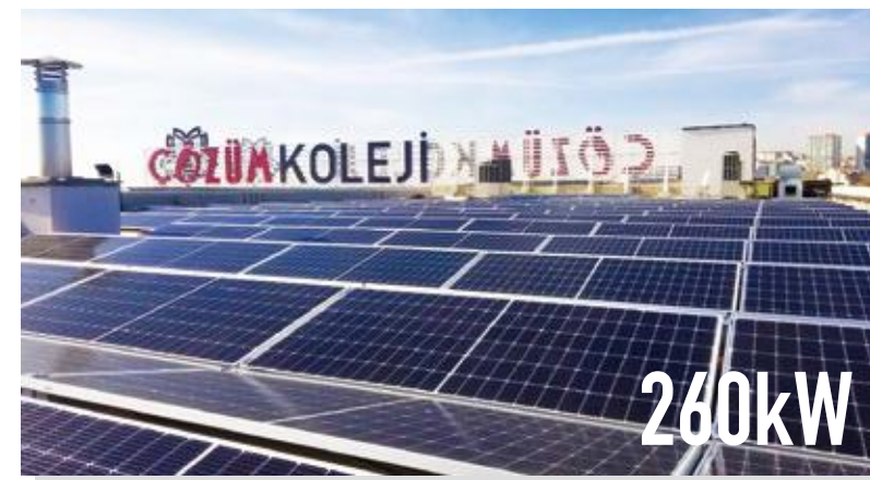
Project Type: Commercial Rooftop Location: Turkey / Ankara Commission Date: 2021-11 Product: SRP-450-BMA-HV
